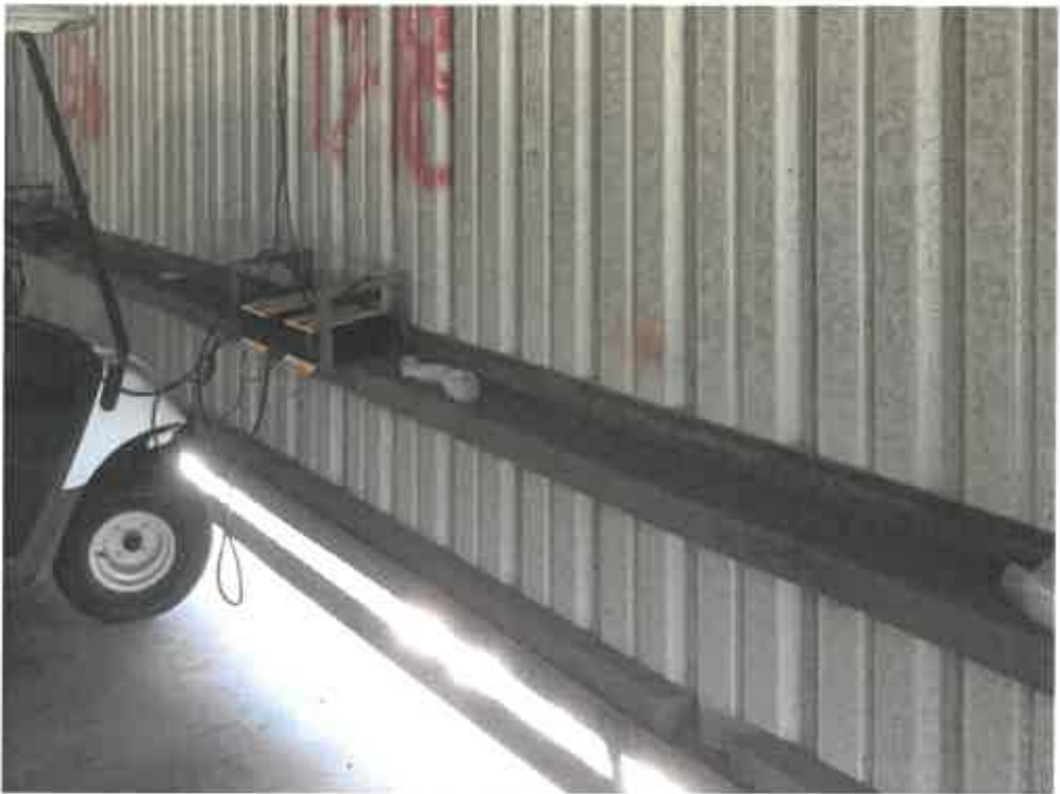
Photo 06 - Rogers Park Golf Course Cart Barn Typical Cladding Interior
