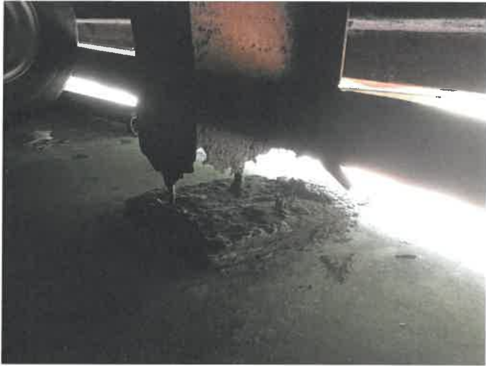
Photo 09 - Rogers Park Golf Course Cart Barn Typical Column with Severe Corrosion
