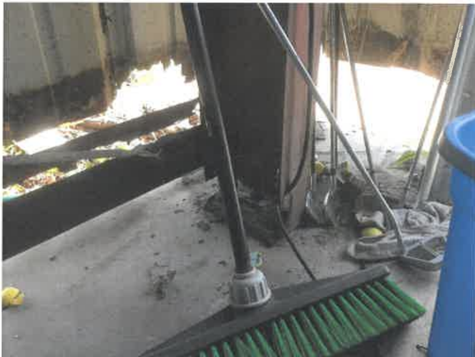
Photo 10 - Rogers Park Golf Course Cart Barn Typical Cladding with Severe Corrosion
