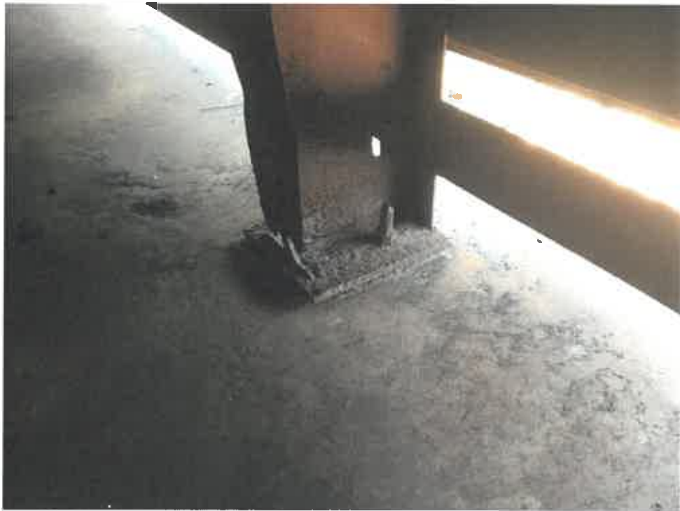
Photo 08 - Rogers Park Golf Course Cart Barn Typical Column with Moderate Corrosion
