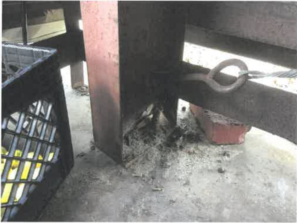
Photo 07 - Rogers Park Golf Course Cart Barn Typical Column with Surface Rust
